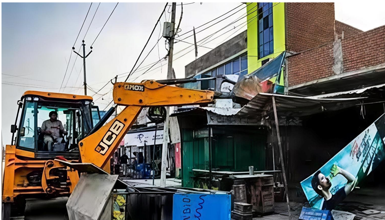
Muhammad Salman's biryani shop demolished in Baheri, Bareilly, Uttar Pradesh.
